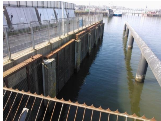
Fig. 23 Current situation at the sieves of cooling system. In the period of floods, the whole area is full of debris and water circulation in cooling system is restricted.
